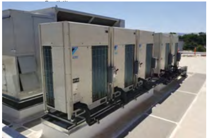
Typical VRF Outdoor Heat-Pump Module
